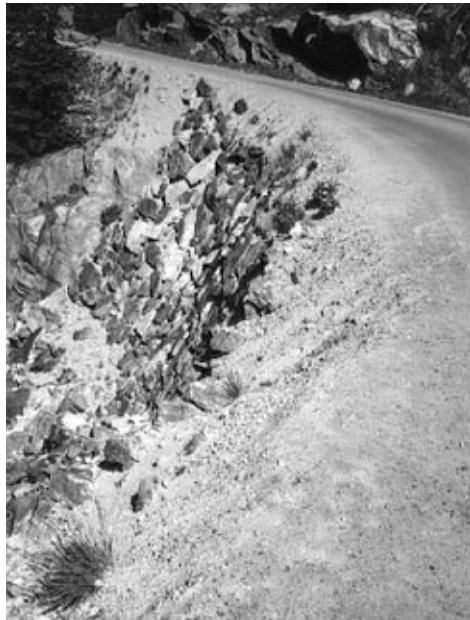
Road bank erosion at Rocky Mountain National Park
