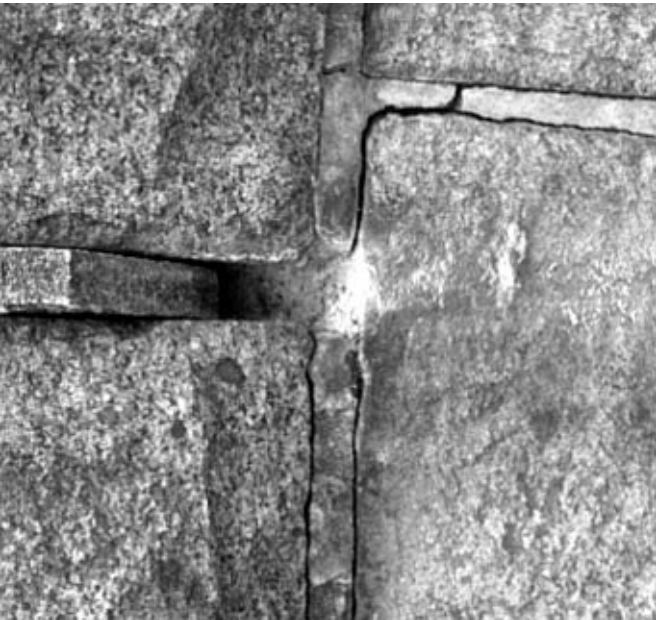
Detail of bridge showing cracks in mortar
