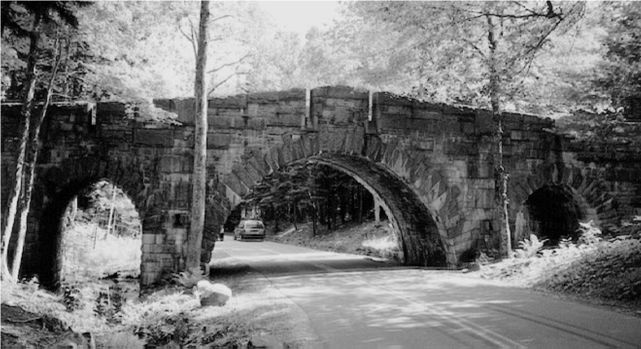
Deteriorating historic bridge at Acadia National Park
