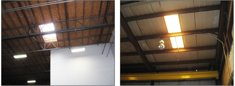
Figure 8: Unsecured Skylights at Industrial Facilities
