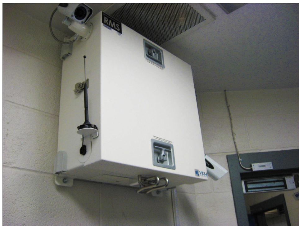
Figure 5: NNSA-Installed Remote Monitoring System
