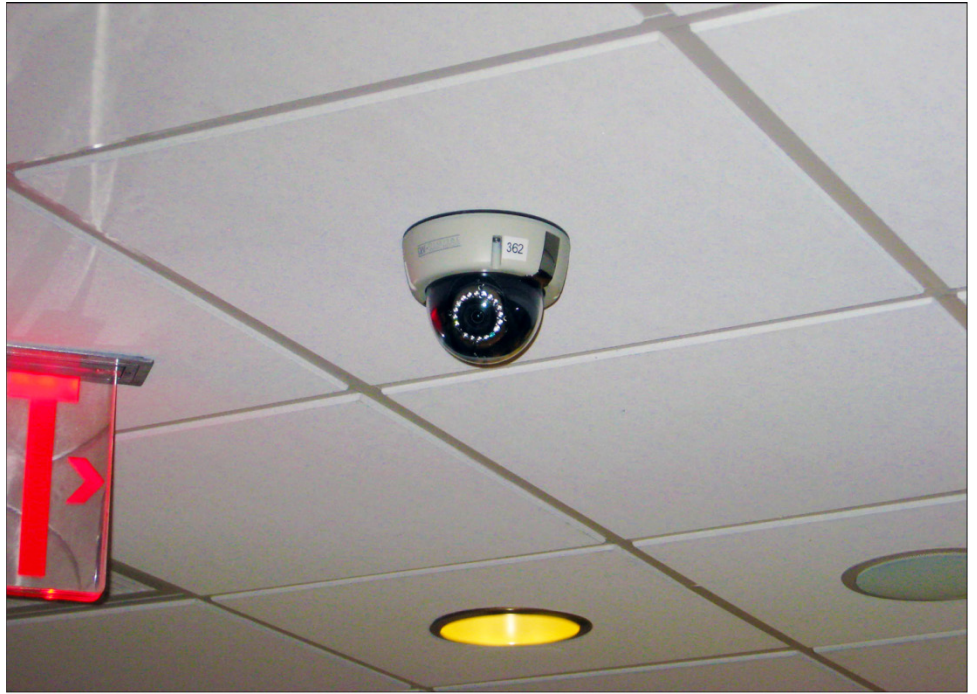
Figure 7: NNSA-Installed Security Camera
