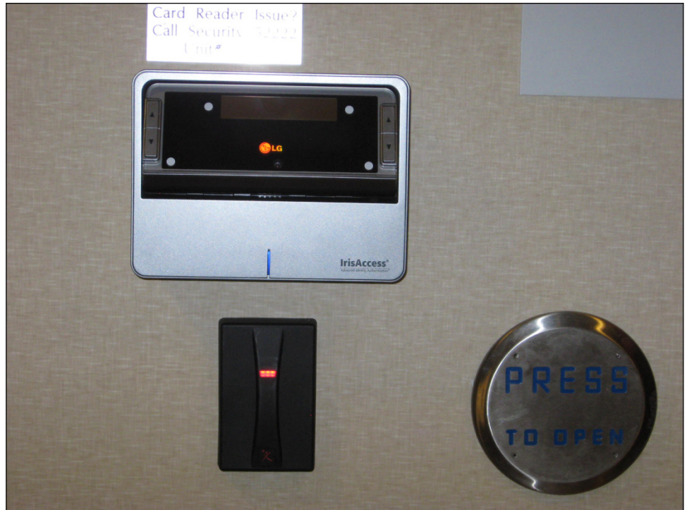
Figure 6: NNSA-Installed Iris Scan with Hospital Card Reader
