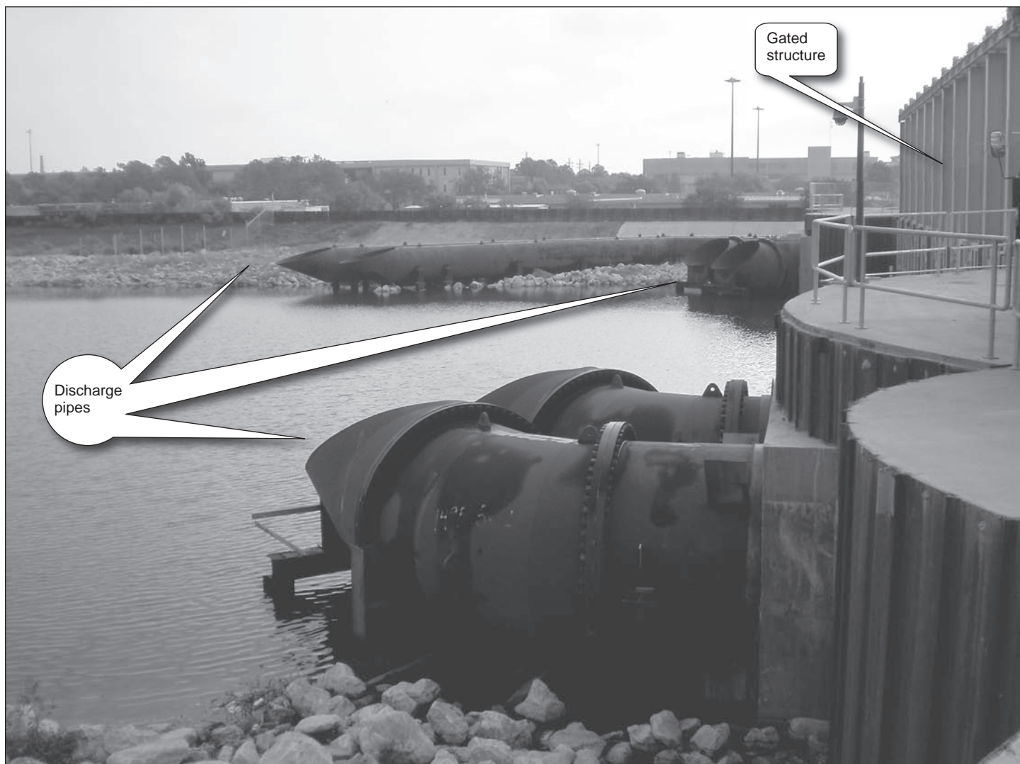
Figure 7: Discharge Pipes at the London Avenue Canal
