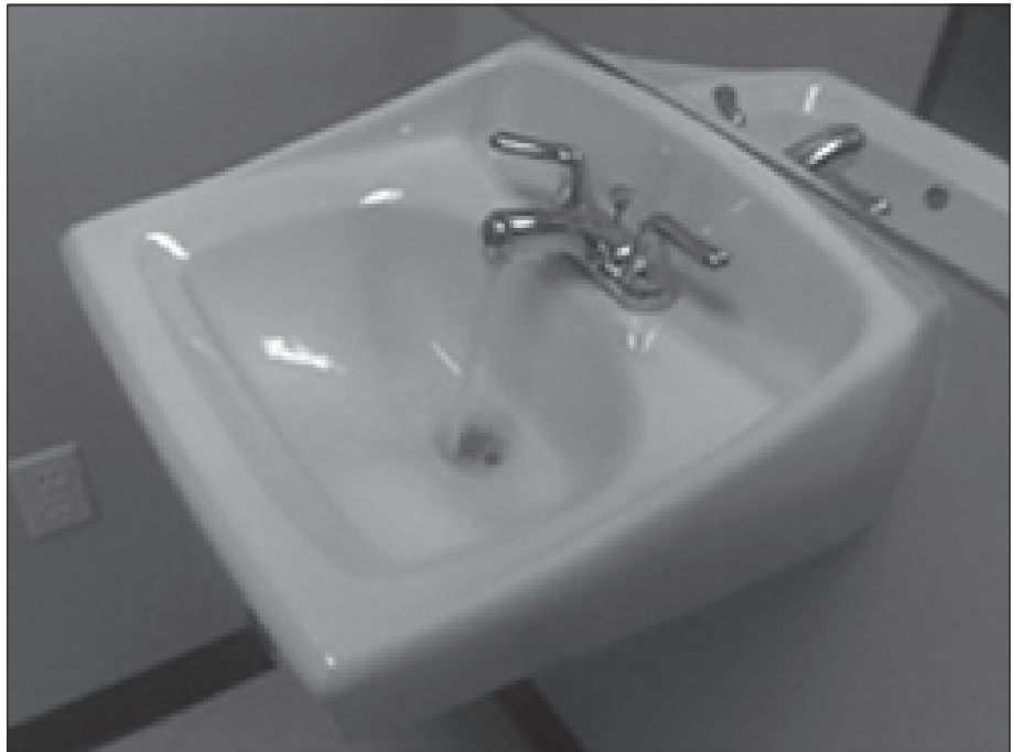
Figure 5: Running Water in the Collection Room in Violation of DOT Protocols
