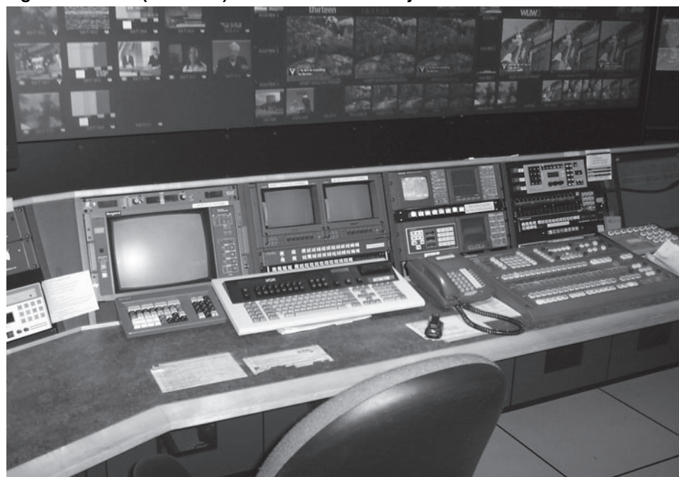
Figure 3: WNET (New York) Master Control Facility
