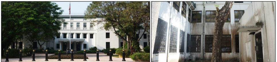
Condition of U.S. Embassy Manila, Philippines – Left: Chancery Office Building; Right: Chancery Courtyard Showing Maintenance Issues, Including Mold and Water Damage
