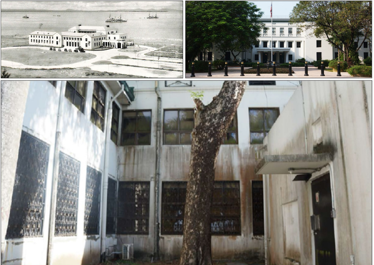
Figure 9: U.S. Embassy Manila, Philippines – Chancery Office Building: Top Left (in 1940); Top Right (in 2019); and Bottom - Chancery Courtyard Showing Maintenance Issues, Including Mold and Water Damage
