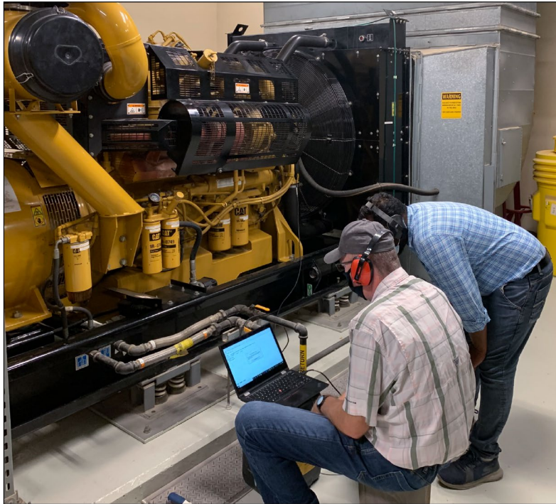
Figure 14: Headquarters-Deployed Technicians Working on a Generator at the U.S. Consulate General Dubai, United Arab Emirates
