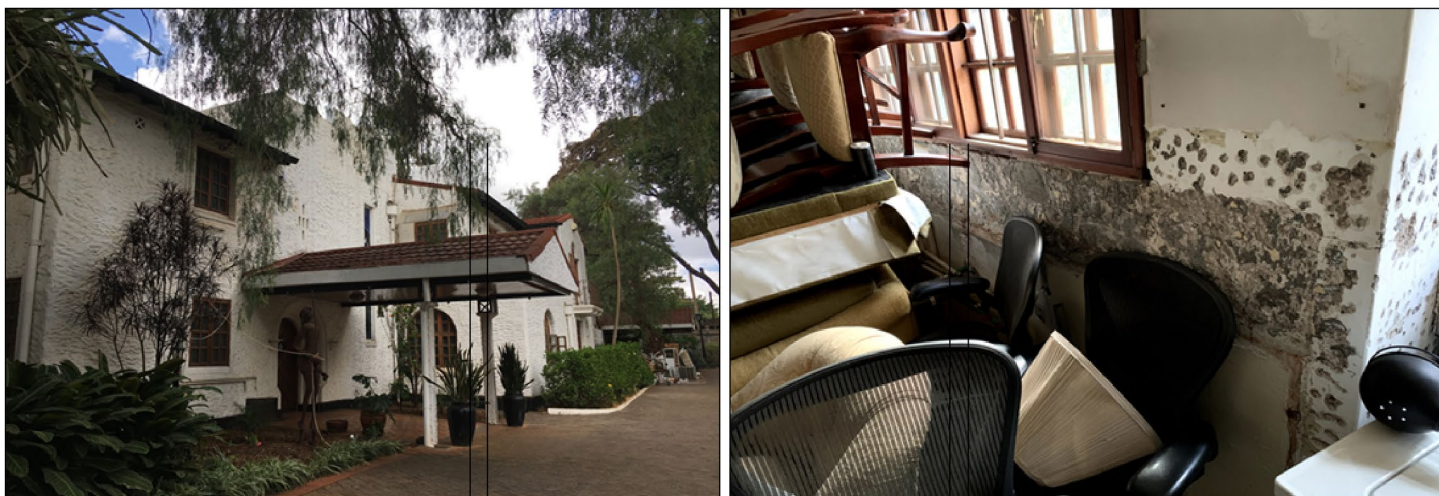
Figure 11: U.S. Ambassadorial Residence - Nairobi, Kenya. Built in 1935. Left - Covered Entryway That Needs to Be Rebuilt. Right – the Kitchen Area Now Demolished and Used to Store Furniture Until State Determines Whether to Rehab the Residence or Replace It Entirely
