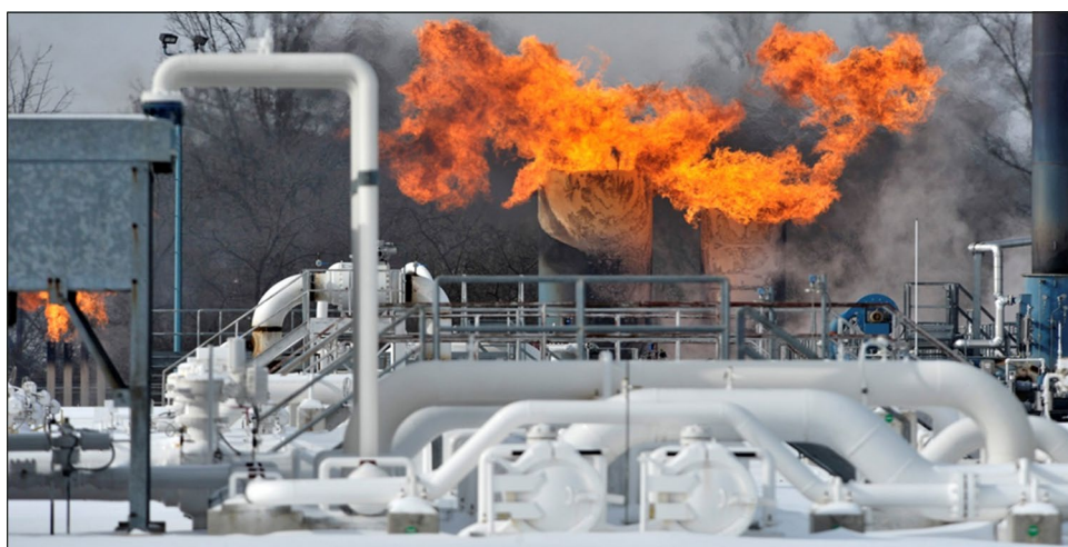
Figure 10: Fire at a Power Facility in Michigan on January 30, 2019
