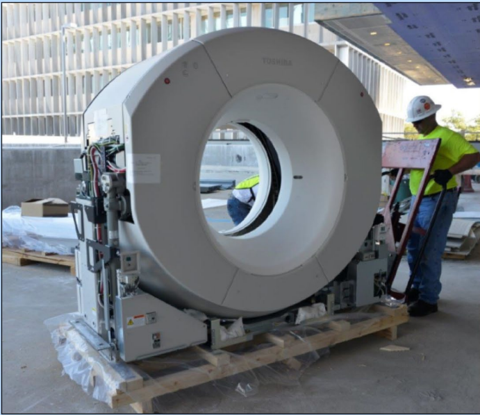
A worker moves a large piece of imaging equipment into a new facility. Installing equipment is a non-recurring activation expense.
