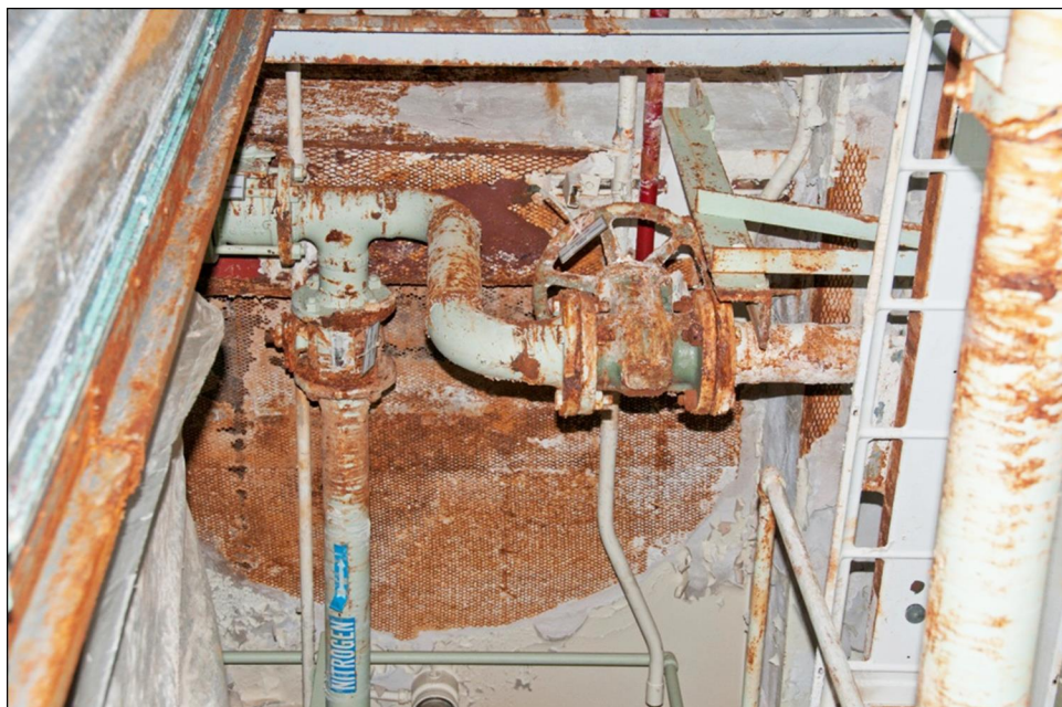
Figure 3: Corroded Equipment in Building 9204-2
